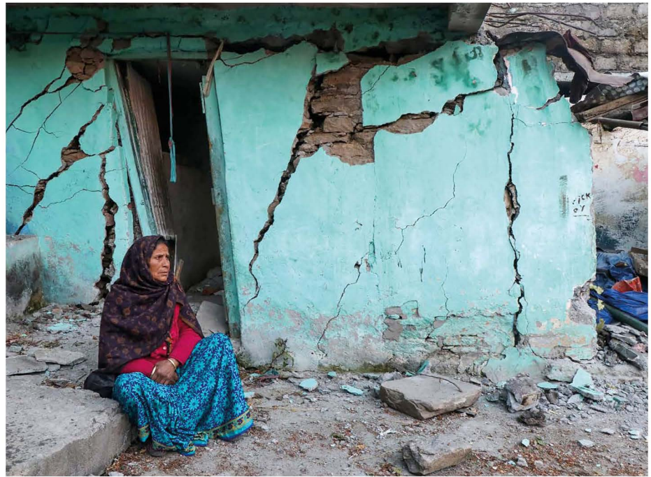
In Joshimath, India, cracks developed in homes in January 2023 as the town began to sink.
