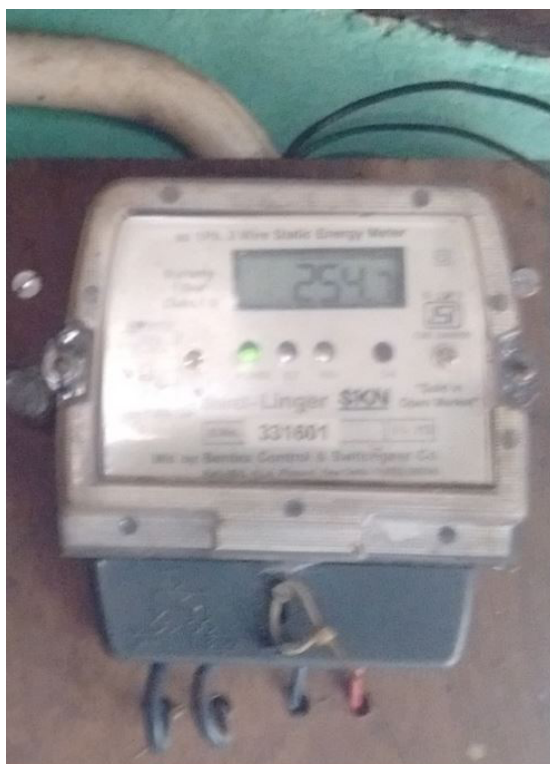
Image 3: The microgrid meter with a straightforward readout of cumulative units consumed.
