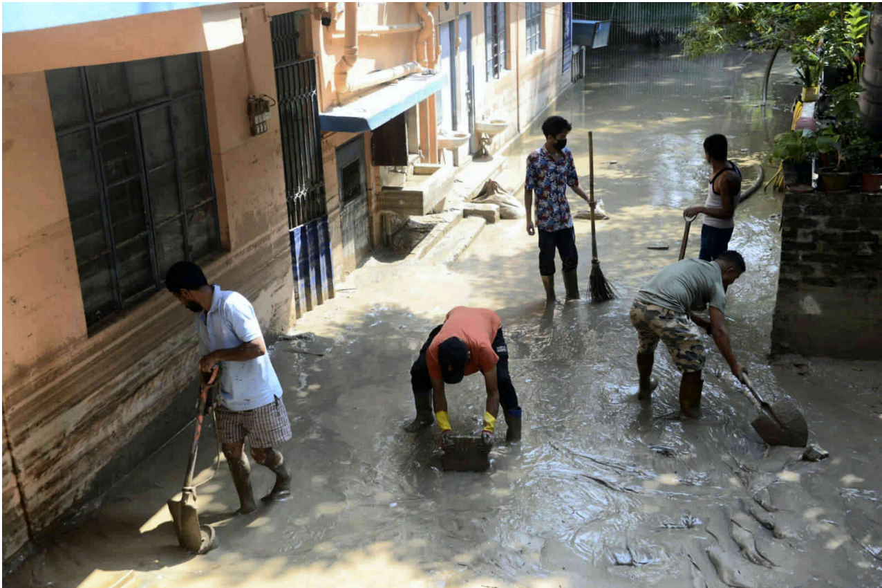
People clear sludge from a road in Pakyong in Sikkim. Credit: PTI.
