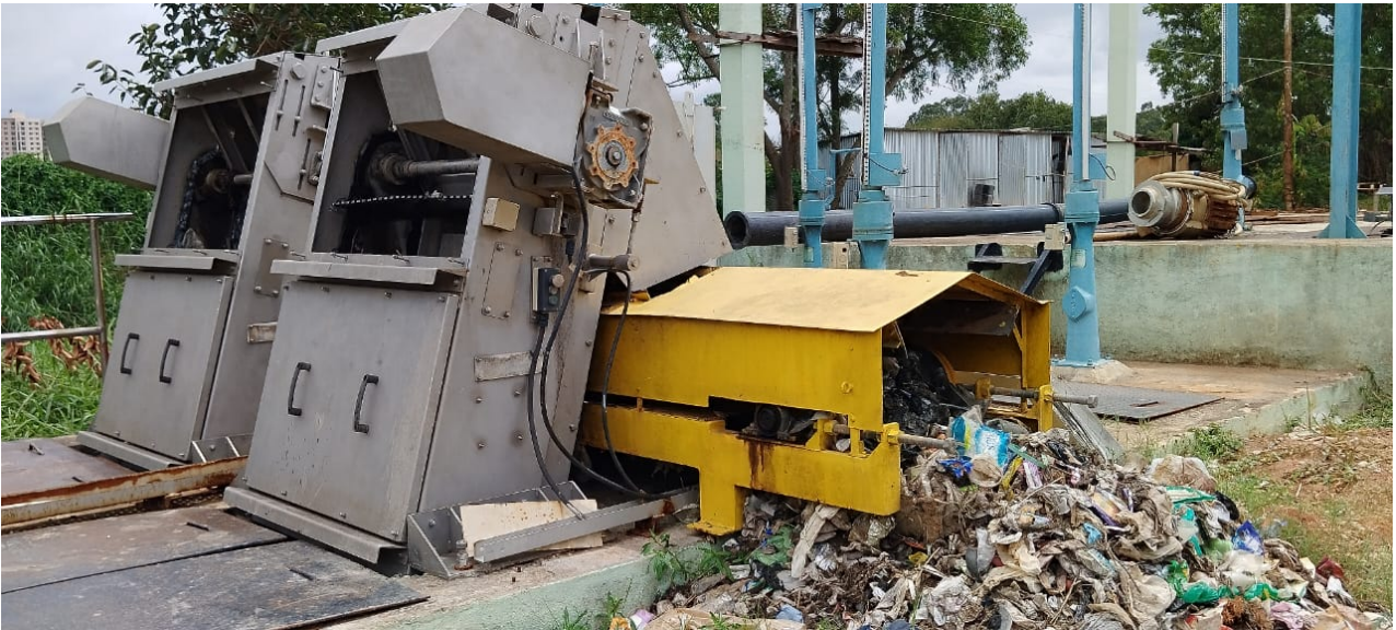
Sludge management at Jakkur Lake (Anshul Rai Sharma)
