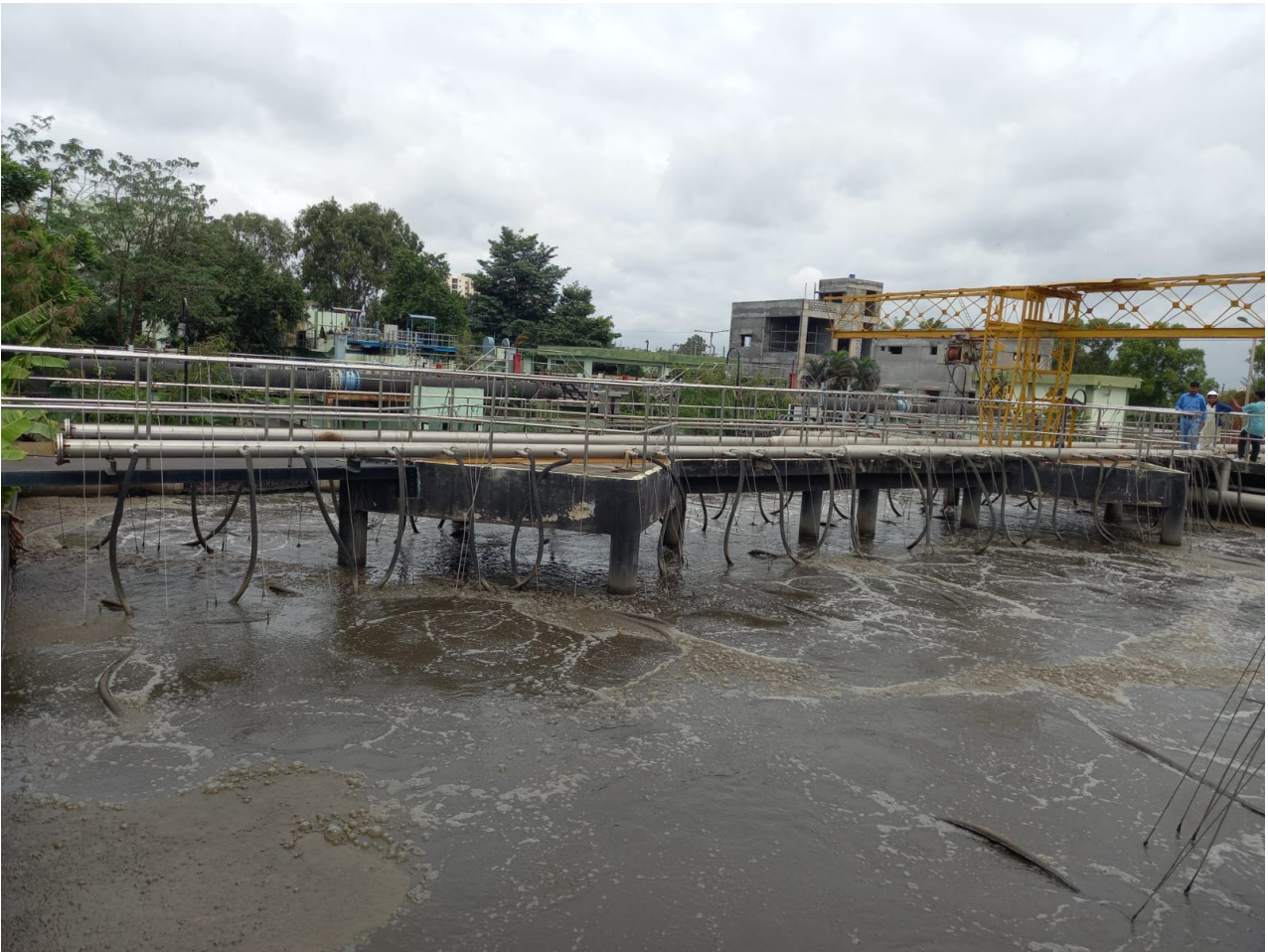
Layered treatment of wastewater at the STP (Image: Anshul Rai Sharma)
