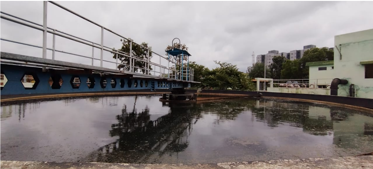
Jakkur Sewage Treatment Plant (Image: Anshul Rai Sharma)
