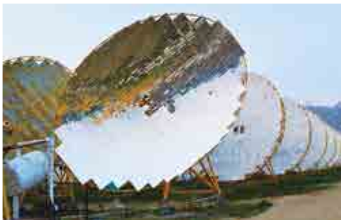
(a) A solar farm.
