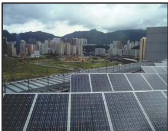
Solar Powerstation in Hong Kong
